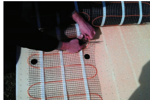
2. At the centre of the mat, cut the mesh - not the cable .
