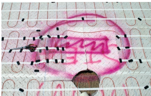
5. Remember to mark goal posts, corner flags, etc. to secure that the heating mat / cables are not damaged when making the holes for the posts.
